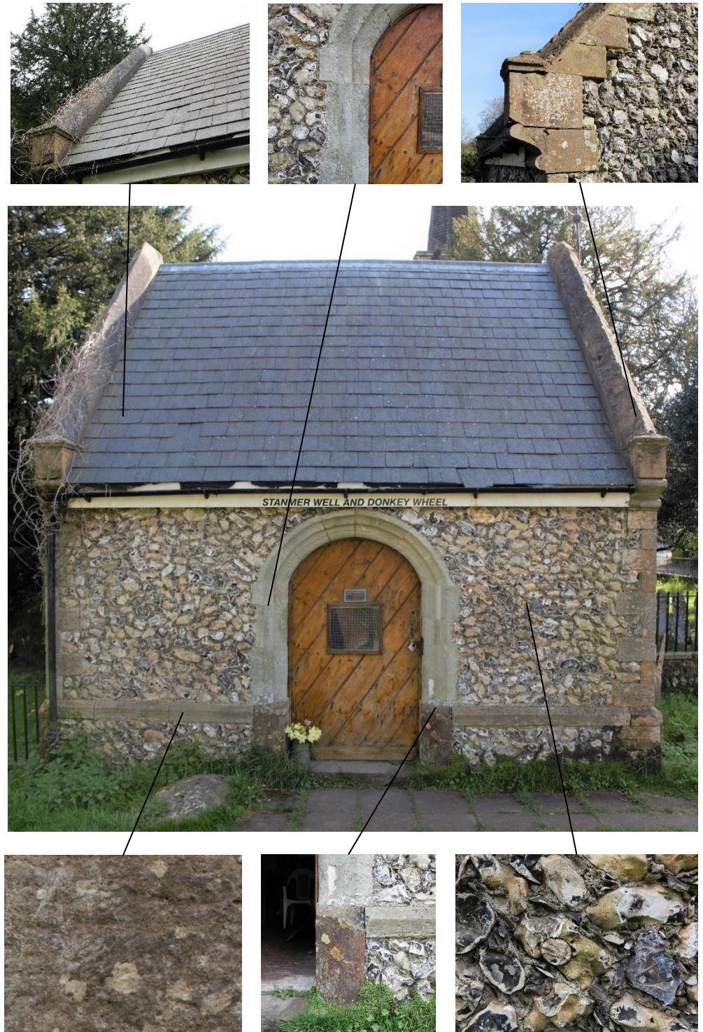
Figure 28: North elevation of well house and various photographs of architectural and material details (Source: Author).
