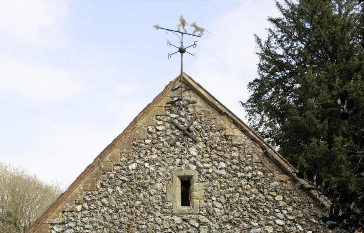
H. Western gable end with coping, chamfered window penetration, metal wall anchor/tie bar and modern weather vane.
