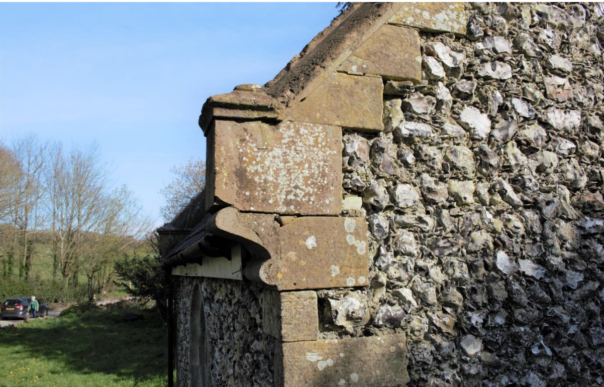
F. Coping, kneeler and corbel with cement repairs - west elevation.
